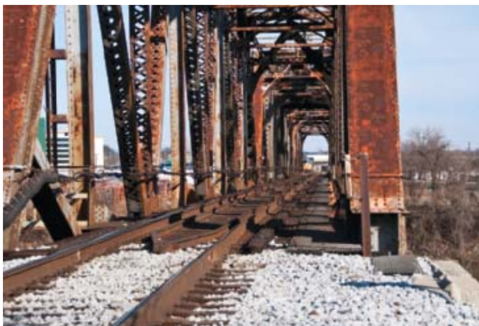
Figure 3.2 The rust that has formed on this bridge is the product of a chemical reaction in which iron and oxygen are the reactants.
