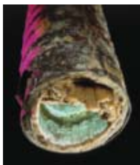
Figure 9.11 The lime scale in this water pipe was caused by hard water.
