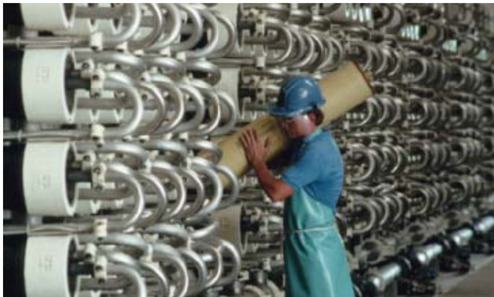
Figure 9.20 High pressure forces water across a semi-permeable membrane inside these vessels. The water that passes through the membranes is completely free of salt and other ions.
